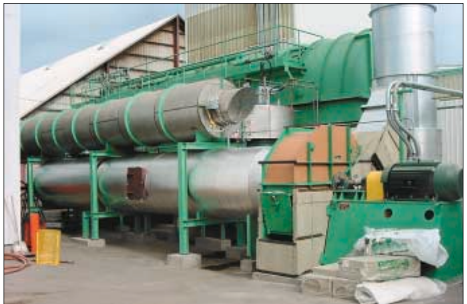
Testing looks good for running the Pro Environmental RTO at LaGrande catalytically.
