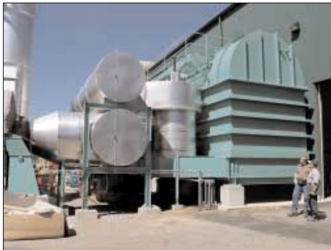
TCO at Elgin saves on gas by operating catalytically at 800° F.
